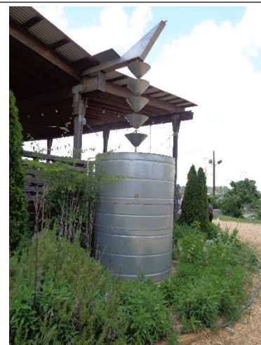
Figure 7.8 Example of rain chain flowing into a Cistern
